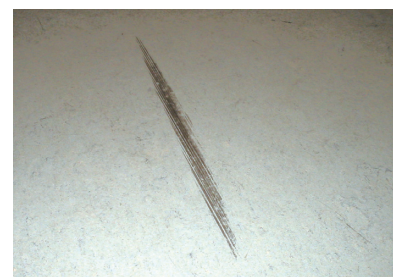
Example of scuff marks by shoes heels, frequently seen in heavy traffic areas.
